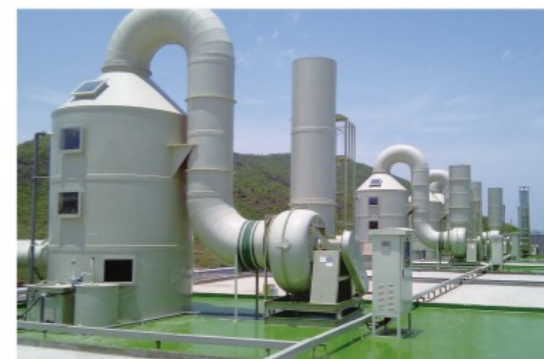
喷淋塔 Spray Tower
