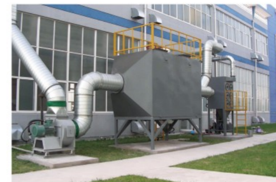
活性炭吸附塔 Activated Carbon Adsorption Tower
